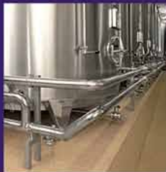
Stainless steel piping
